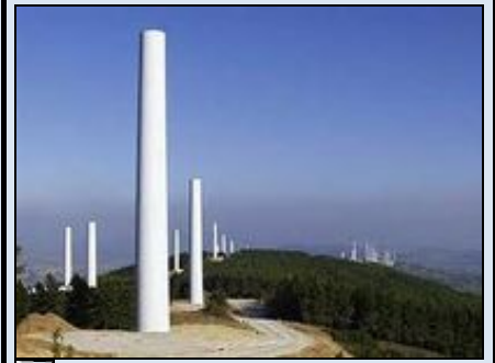
Fig 8(a) Tubular tower
